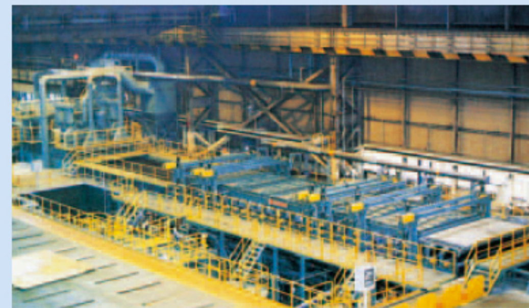
連続酸洗設備/Continuous pickling system
